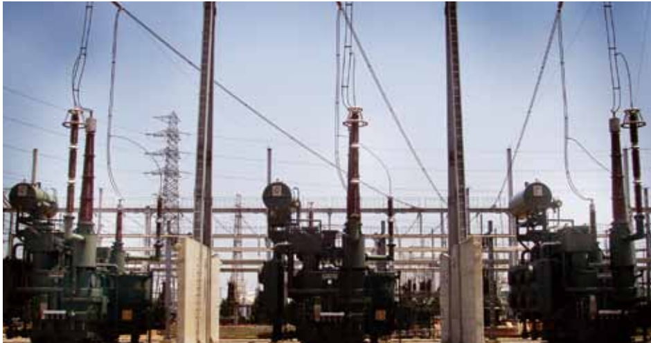
345kV, 500MVA in TPC (Taiwan Power Company)
