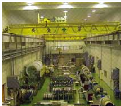
Dual Clean rooms for Coil winding and Internal Assembling
