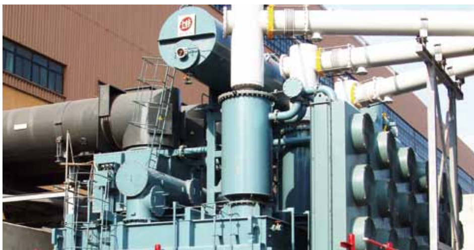
345kV, 650MVA in TPC (Taiwan Power Company)
