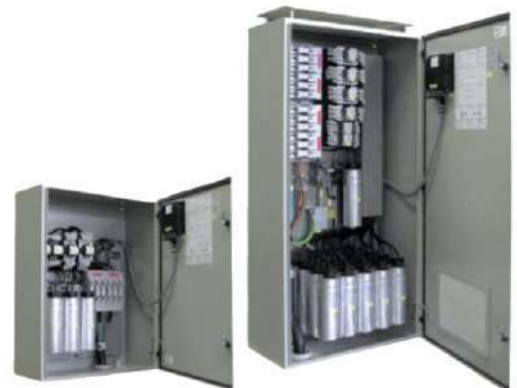
Power Factor Correction System
