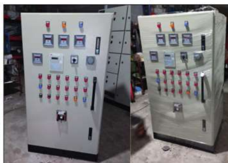
Relay Control Panel SAS Steel Mill
