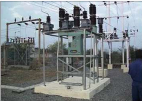
33KV1250A Outdoor type VCB Safiul Alam Steel Mills Ltd.
