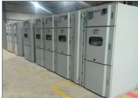
11KV 1250/630A HT Switchgear Panel Narayanganj Wasa
