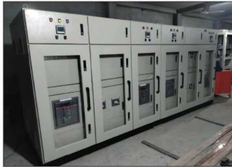
Main Distribution Board (MDB) Metrocem Ispat Ltd.
