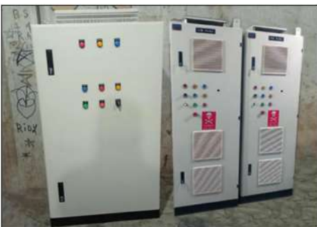
Saidabad Water Treatment Plant 450KW VFD Panel
