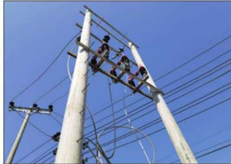
33KV 1250A ABS with Earth Switch Danga Industrial Park at Narsingdi
