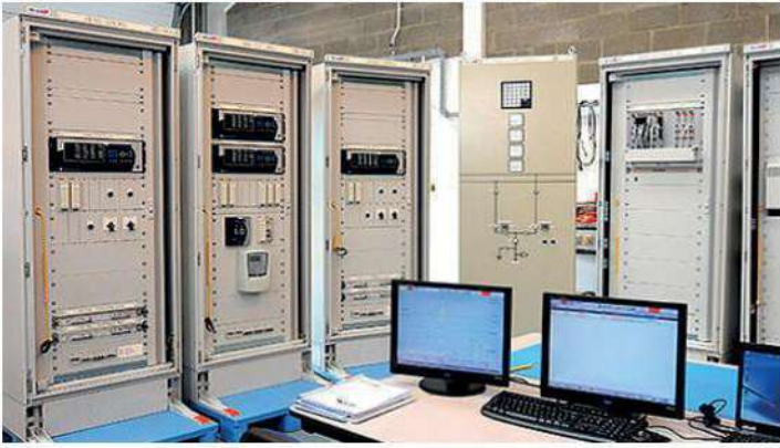
Industrial Substation Automation
