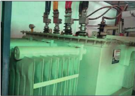
11/0.415 KV 1250 KVA Sub-Station Medicon Pharmaceuticals Ltd.
