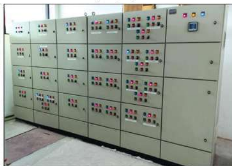
Low Voltage MCC Panel Far East Group
