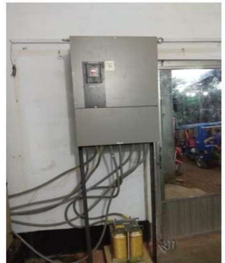
CNG Station 260kW Hitachi Inverter
