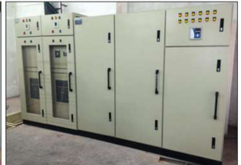
LT & 1200KVAR PFI Plant Naheed Group
