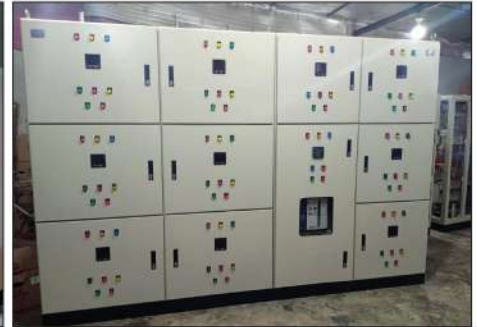
Motor Control Center (MCC) FKL Spinning Ltd.
