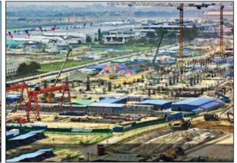
Low Voltage Equipment Hazrat Shahjalal International Airport Terminal-3
