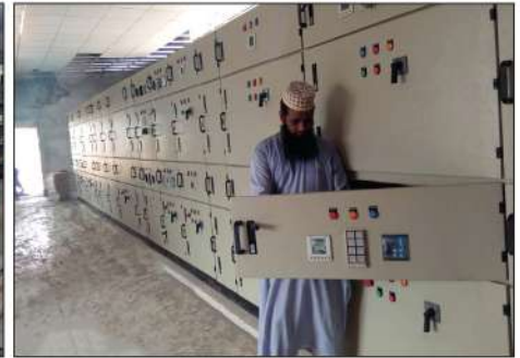
Low Voltage Switchgear with Bus-coupler Pretty Composite Textiles Industries Ltd.
