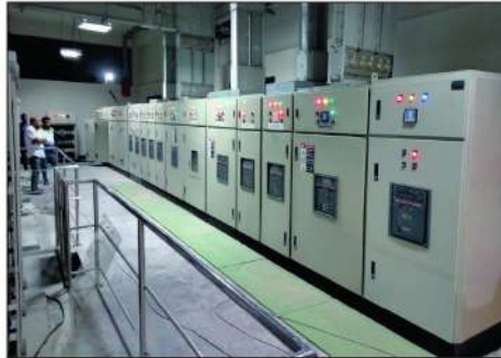
Low Voltage Switchgear Far East Spinning Industries Ltd.
