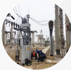
SUBSTATION CIRCUIT BREAKER
